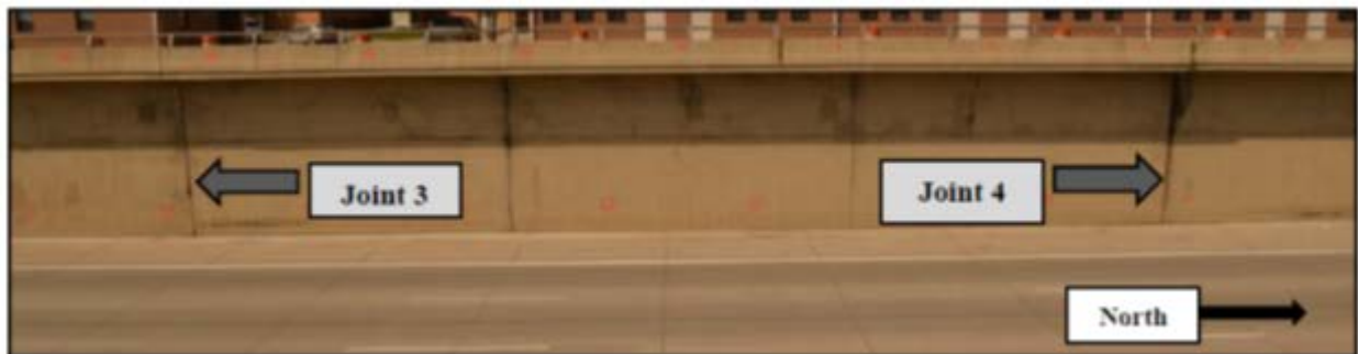
Figure 21: Individual retaining wall sections and joints between them, at the M-10 test location
